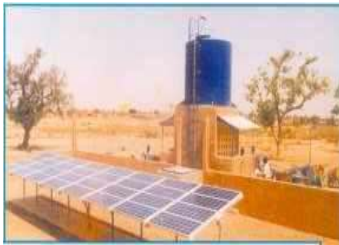
Pumping station with sunpower
