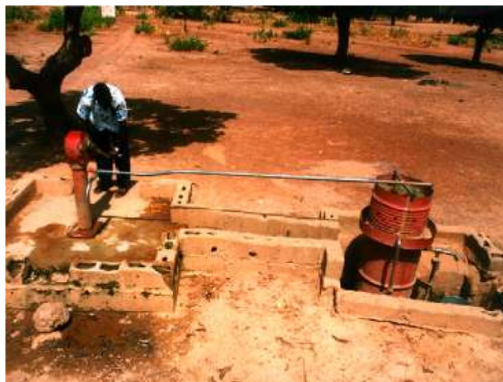
AF iron removing unit
