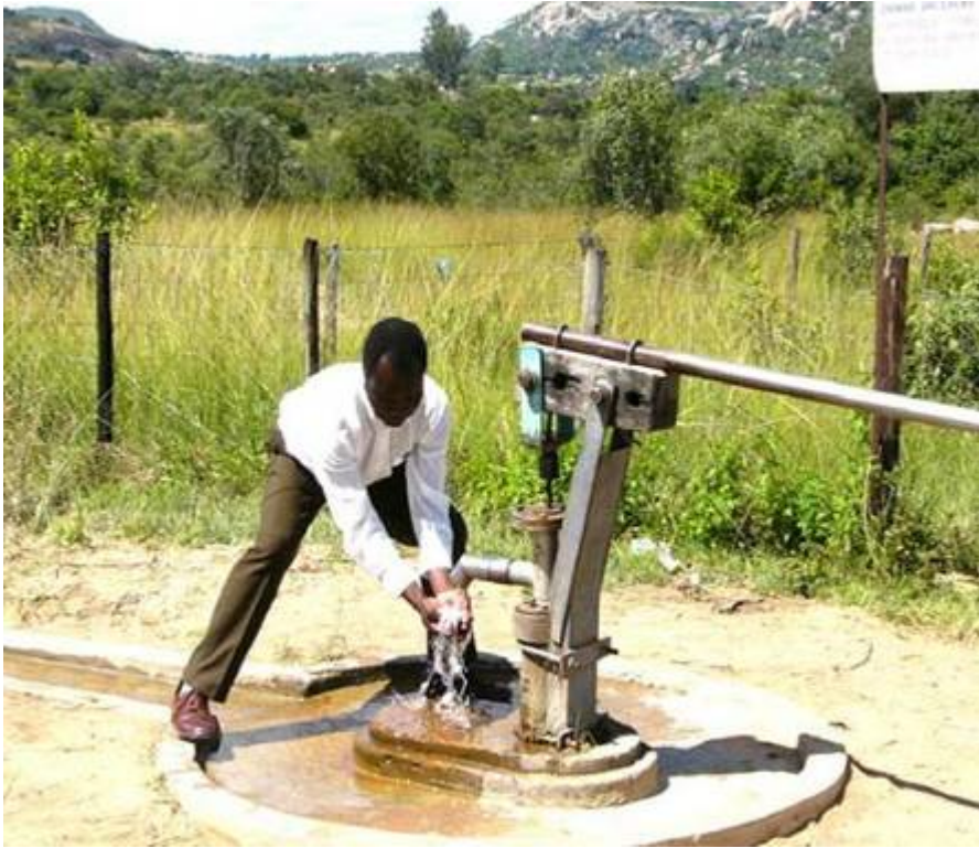
Figure 6: bush pump in Murehwa district; the sign board indicates that doing the laundry and watering cattle are prohibited.
