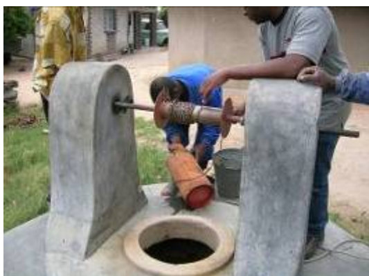
Figure 2: A typical upgraded family well with windlass and bucket in Marondera district
